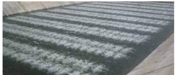
EJIP WWTP (Indonesia)
